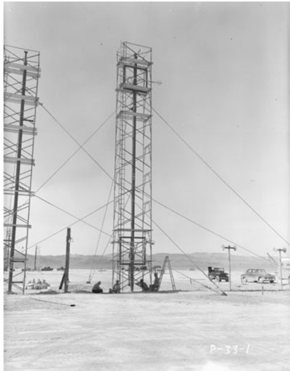
Tower for thermal instrumentation with scaffolding, Station 206
